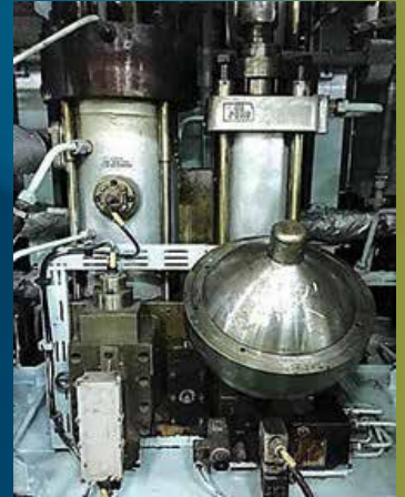
Hydraulic Cylinder Unit (HCU)
